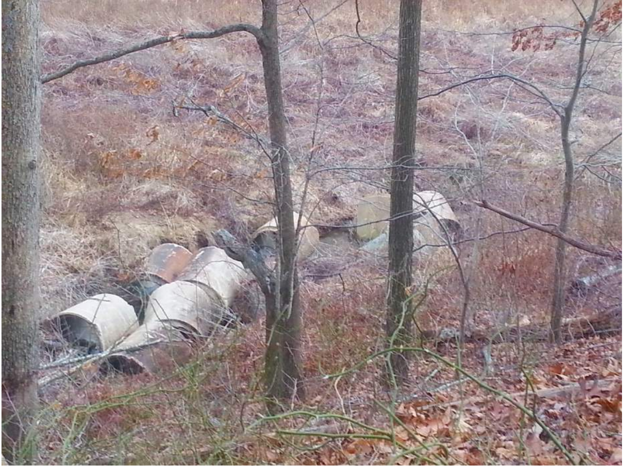
Concrete sectional pipes used to bridge the small creek shown in 2002 aerial right hand side at lower part of Triadelphia Rd approaching Triadelphia from Howard County. Likely late 19 th -early 20 th century. May have been used in Triadelphia Rd rebuild after 1889 massive flood.
