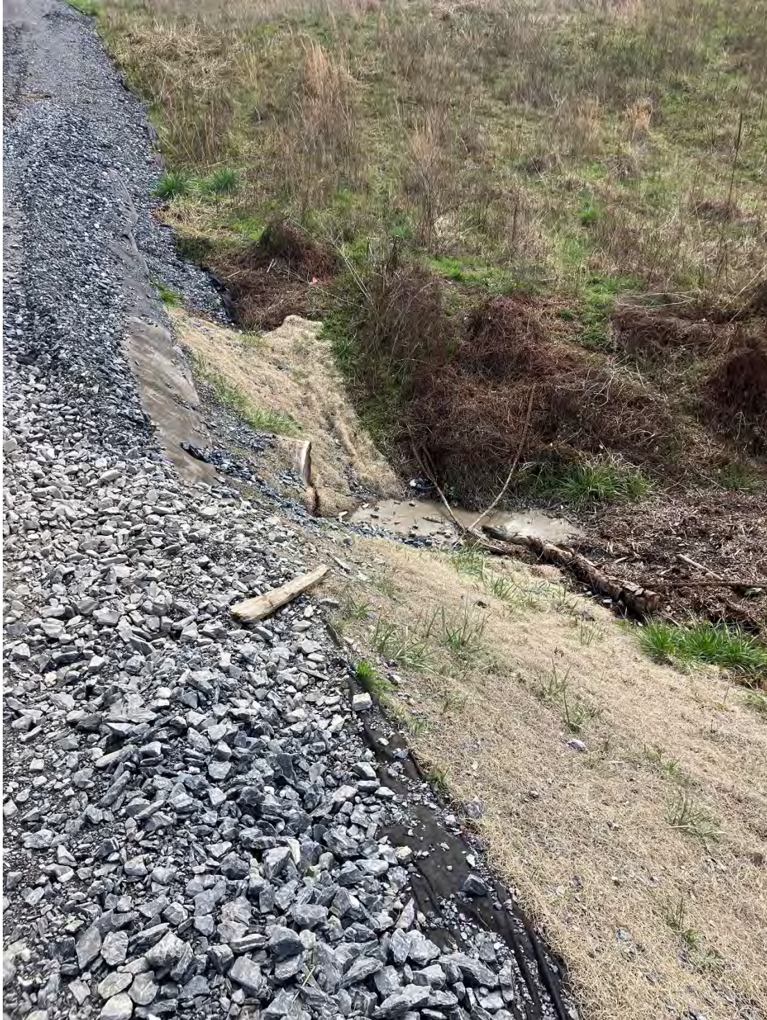
Figure A: There were issues found with a lack of sediment and erosion controls on the edge of the access road off of the Mouth of the Monocacy Road. Sediment pollution was noticed in the waterways (Waters of the State) that are crossed by the access road leading to the boring operation. Sediment pollution remains in a position likely to pollute the Waters of the State.
