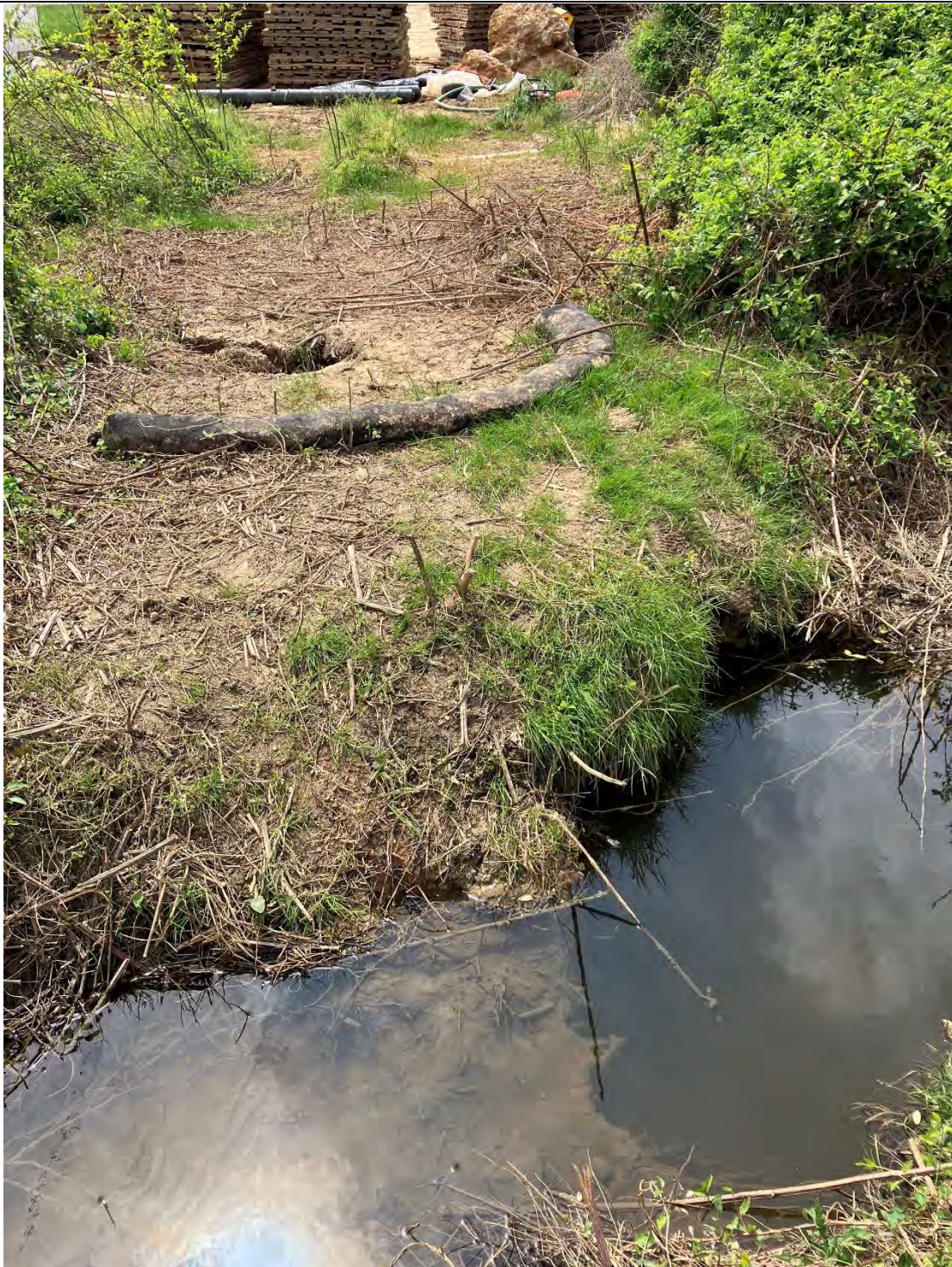
Figure G: There were cracks/fractures in the ground, noticed at the frac-out location in Segment 16 (located at roughly 39.3158900, -77.4996900). This frac-out has been cleaned up but the cracks/fractures have not been stabilized. Sediment (bentonite) pollution has occurred in the Waters of the State but was contained during the time of the inspection.
