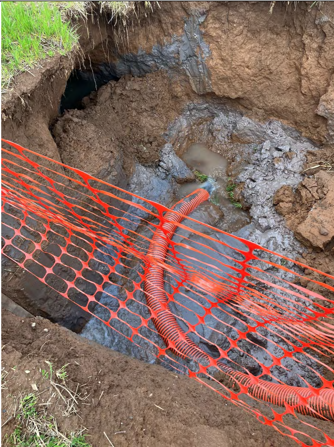
Figure C: There was a frac-out within a previously bored hole that was later abandoned. This location was outside the LOD. Also, sediment-laden water is being pumped out of the other frac-out locations to this abandoned bored hole. Sediment (bentonite) pollution was found in the Waters of the State and remains in a condition likely to continue to pollute.
