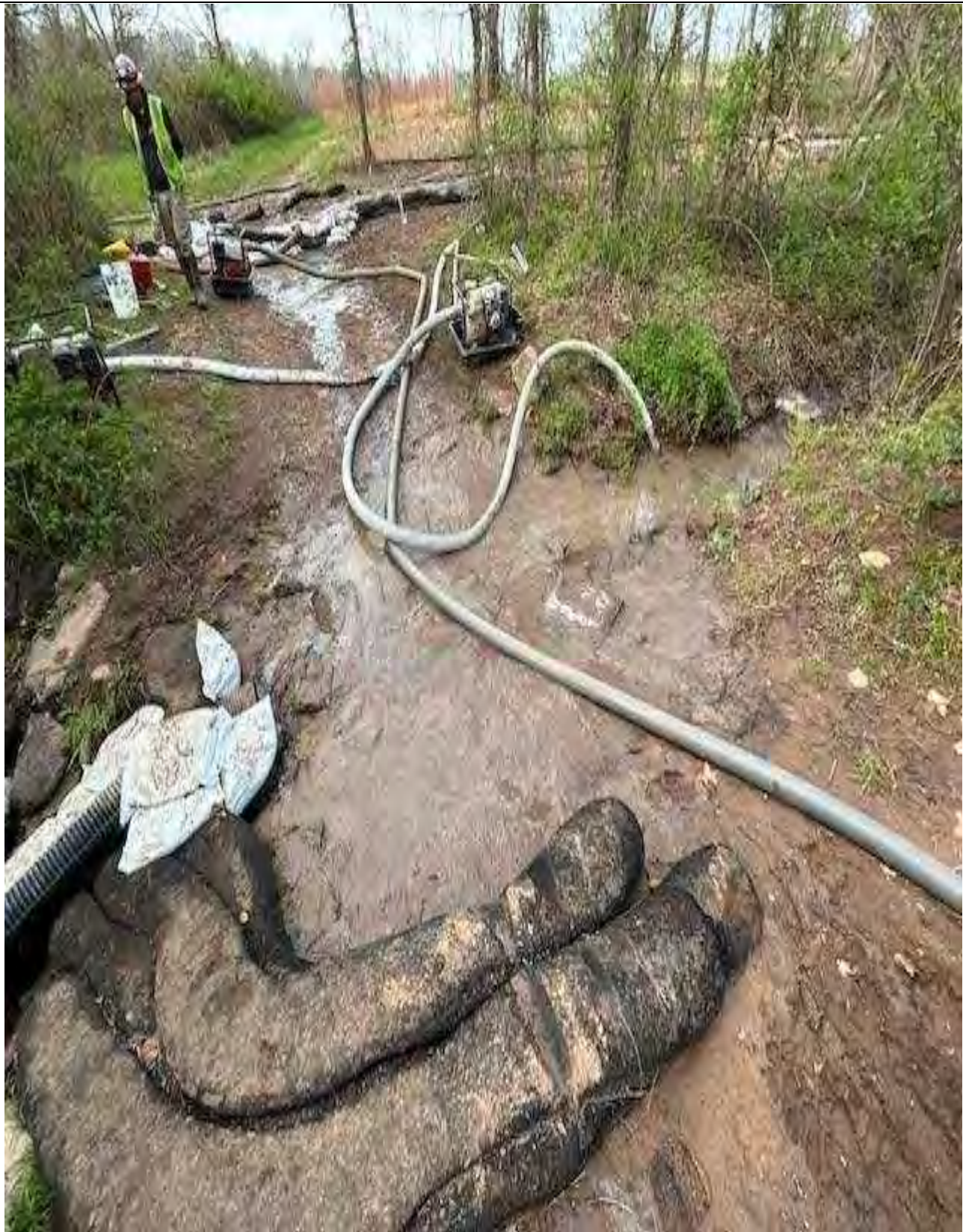
Figure J: "Pumping and dam area downstream. Dewatering pools present in the distance." The photo was taken on 04/08/2024 by Douglas Cochran with Frederick County Government.
