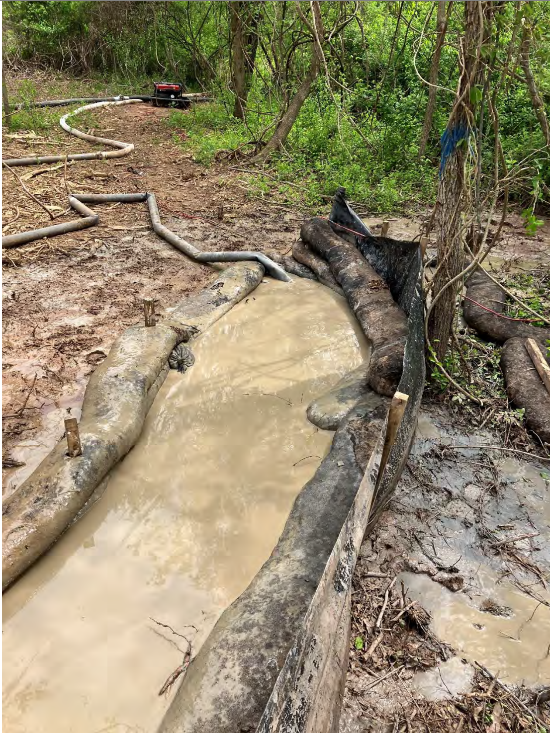
Figure A: One of the undocumented frac-outs was found by the documented (in the 04/10/2024 MDE inspection report) frac-out on the western side of the waterway (UT to Monocacy River, use class I-P waters), on dry land. This frac-out is located at Segment 2. Sediment (bentonite) pollution is occurring in the Waters of the State but is contained at a downstream point.
