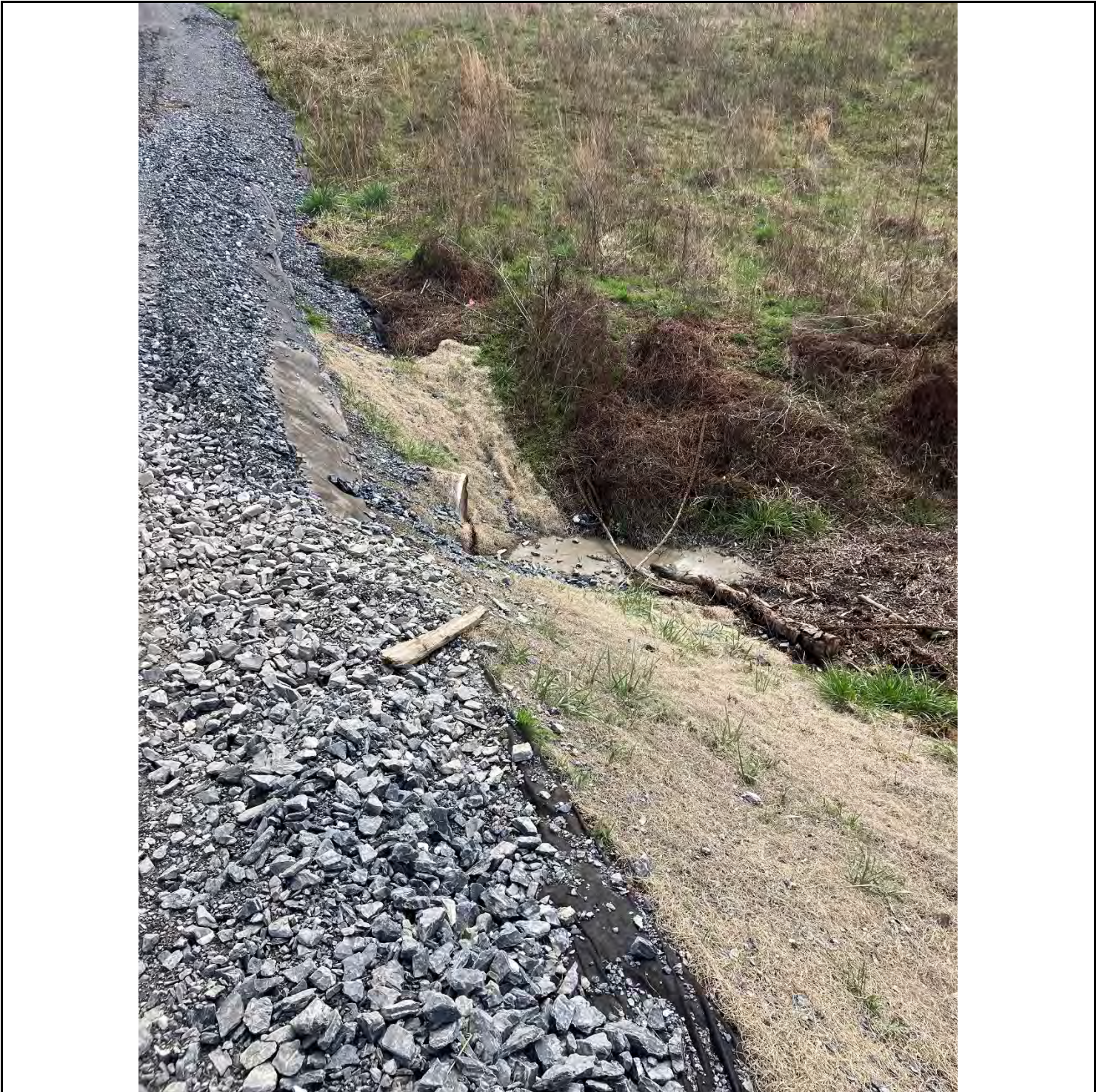
Figure A: There were issues found with a lack of sediment and erosion controls on the edge of the access road off of the Mouth of the Monocacy Road. Sediment pollution was noticed in the waterways (Waters of the State) that are crossed by the access road leading to the boring operation. Sediment pollution remains in a position likely to pollute the Waters of the State.
