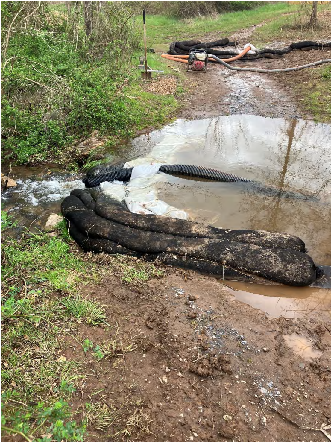
Figure F: The clear water diversion appeared to be discharging clear water and down stream of the frac-out locations were found to be clear during the time of the inspection.
