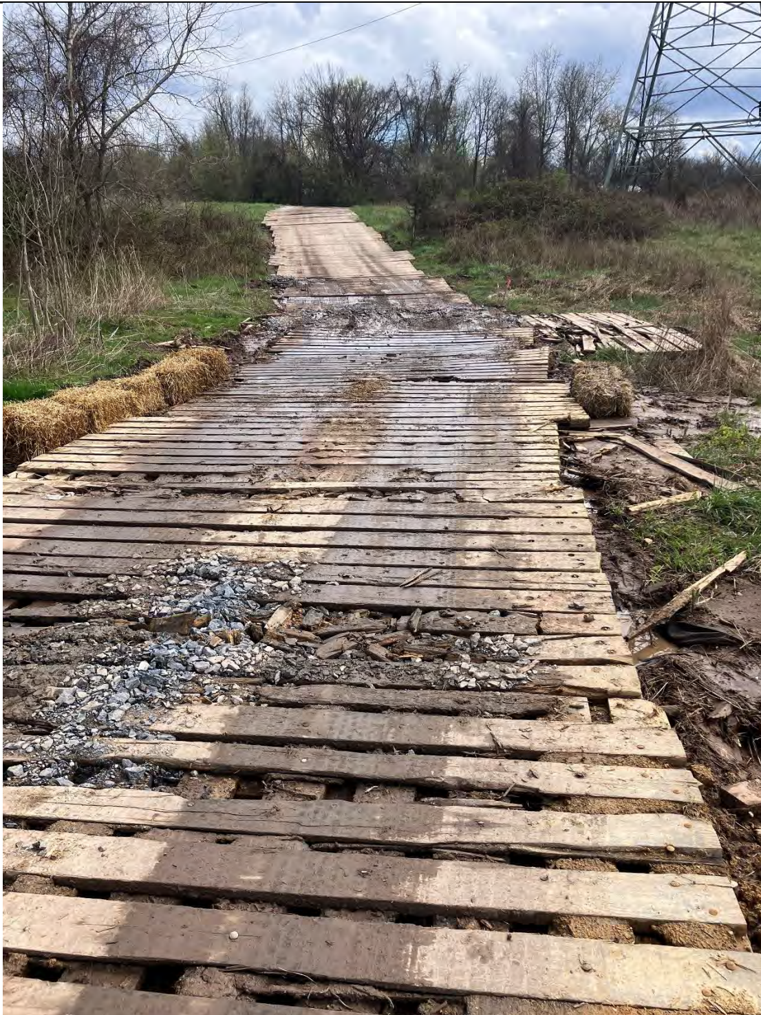
Figure B: There were issues found with the sediment and erosion controls on the access road off of the Mouth of the Monocacy Road. The matting was crushed in some locations and/or sinking. Crossed waterways and wetlands lacked adequate controls at the edge of the matting. Sediment pollution was noticed in the waterways (Waters of the State) that are crossed by the access road leading to the boring operation. Sediment pollution remains in a position likely to pollute the Waters of the State.
