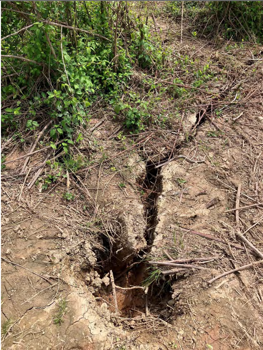
Figure F: There were cracks/fractures in the ground, noticed at the frac-out location in Segment 16 (located at roughly 39.3158900, -77.4996900). Sediment (bentonite) pollution has occurred in the Waters of the State but was contained during the time of the inspection.
