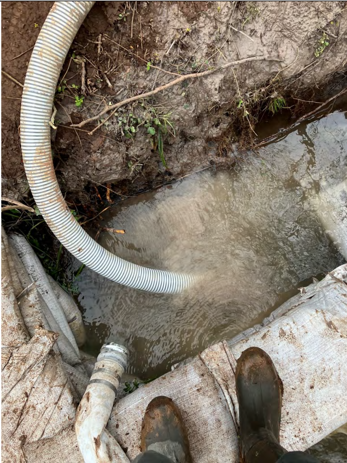
Figure D: Another frac-out was within the channel of a waterway (UT to Monocacy River, use class I-P waters), and the discharge point was located underwater; it was evident that there was sediment-laden water discharging into the waterway. A sandbag containment was set up within the waterway to contain the sediment-laden discharge and to pump out the discharge water to the abandoned borehole (where there was also frac-out discharge). Sediment (bentonite) pollution was found in the Waters of the State and remains in a condition likely to continue to pollute.
