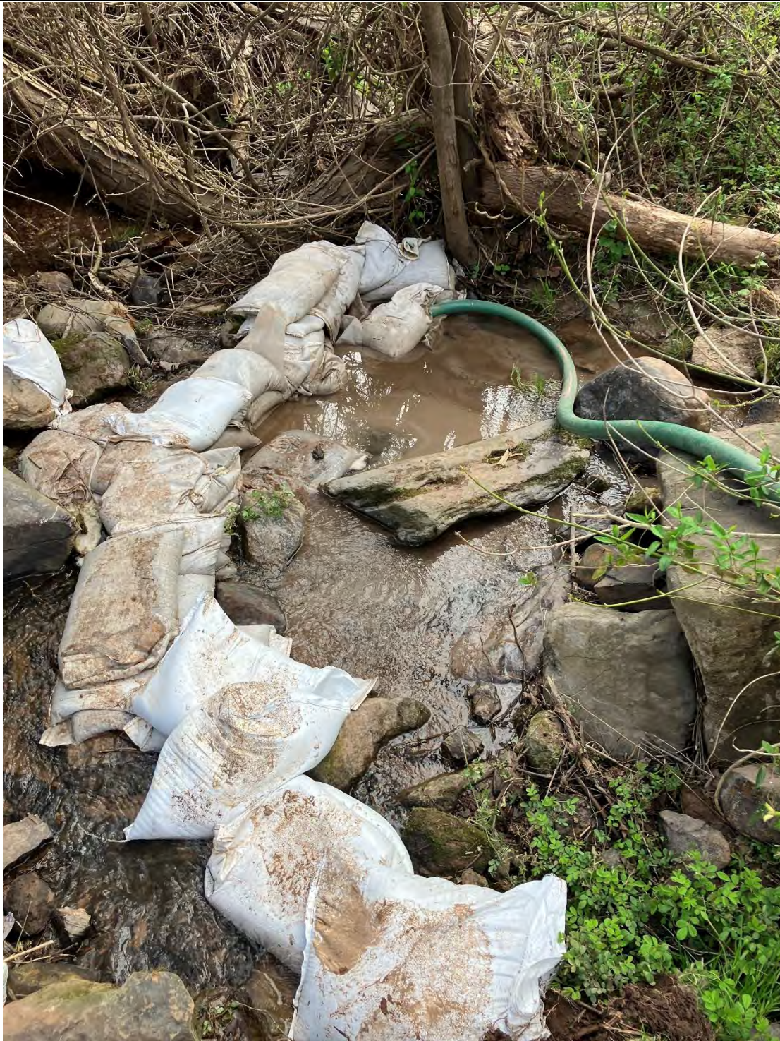
Figure C: There was another frac-out found within the channel of the waterway (UT to Monocacy River, use class I-P waters) just downstream where the farm stream crossing is located; there was sediment deposition deposited in the stream where the frac-out occurred. All of the frac-outs that occurred in the waterway (UT to Monocacy River, use class I-P waters) had sandbag containments around the discharge points. Sediment (bentonite) pollution was found in the Waters of the State and remains in a condition likely to continue to pollute.
