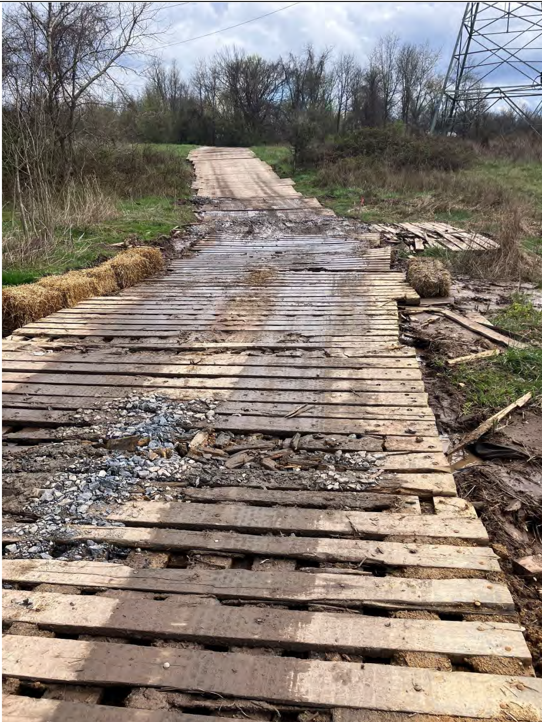
Figure B: There were issues found with the sediment and erosion controls on the access road off of the Mouth of the Monocacy Road. The matting was crushed in some locations and/or sinking. Crossed waterways and wetlands lacked adequate controls at the edge of the matting. Sediment pollution was noticed in the waterways (Waters of the State) that are crossed by the access road leading to the boring operation. Sediment pollution remains in a position likely to pollute the Waters of the State.
