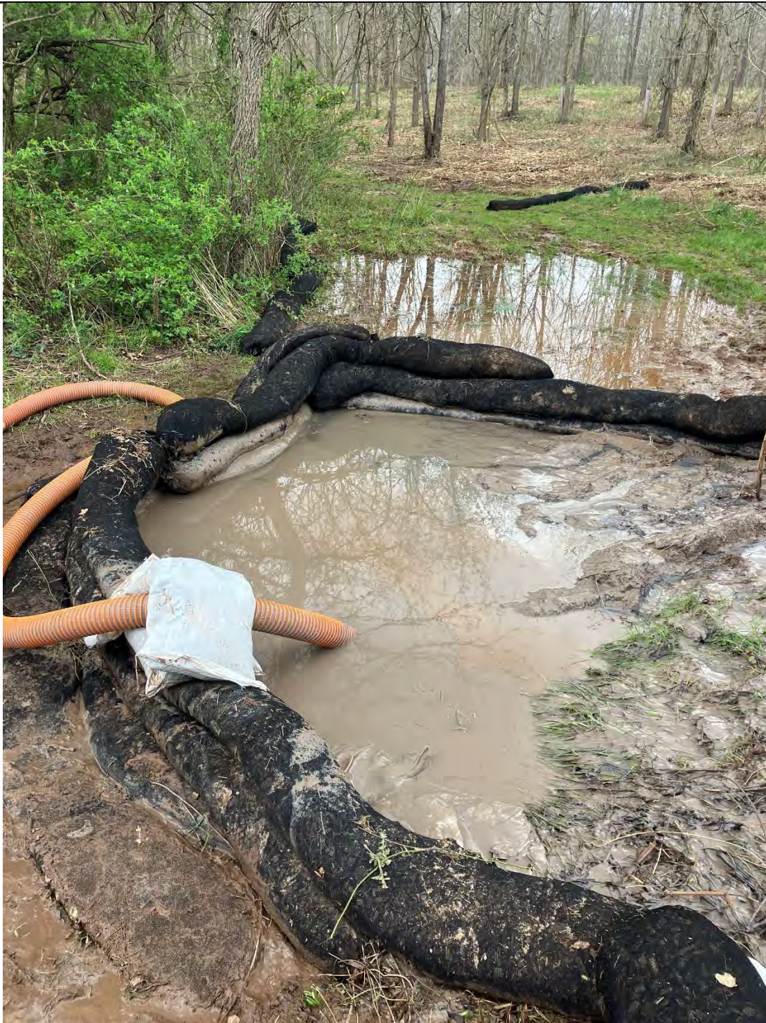
Figure E: The other frac-out was on the western side of the same waterway but the frac-out was on dry land and contained with filter logs; this frac-out was being pumped out. Sediment (bentonite) pollution was found in the Waters of the State and remains in a condition likely to continue to pollute.
