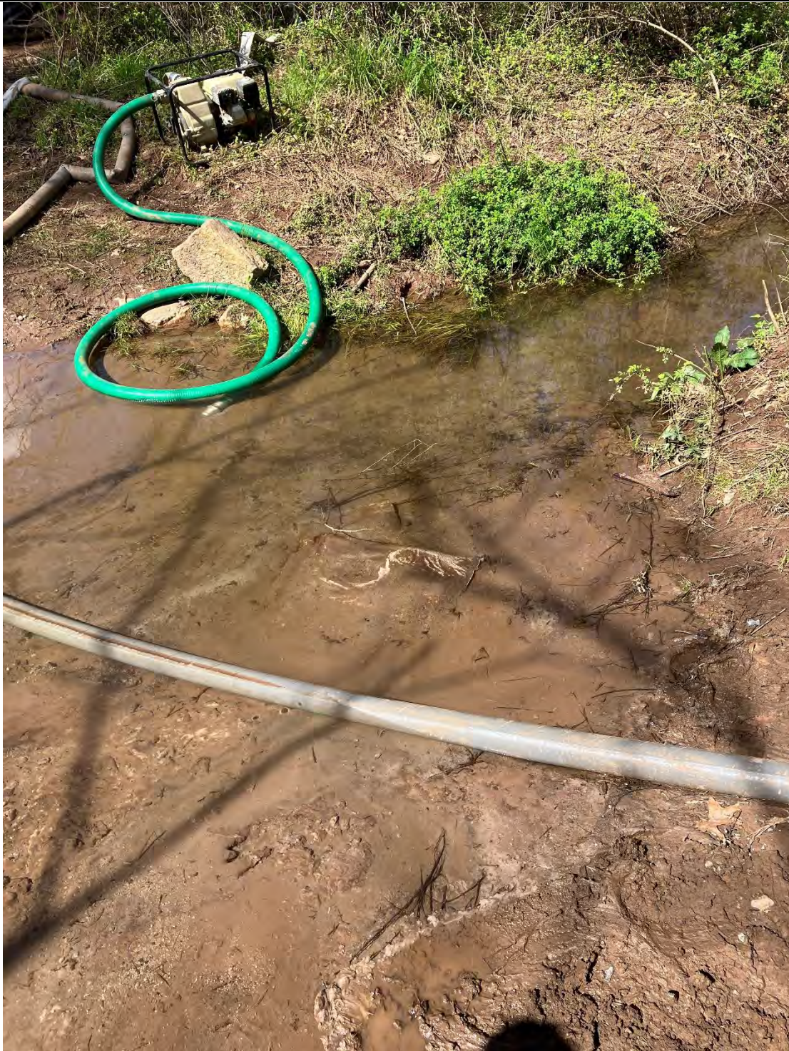
Figure G: Sediment pollution was found in the Waters of the State where the farm waterway crossing is located. There was substantial sediment (bentonite) pollution downstream of where the frac-outs were located.
