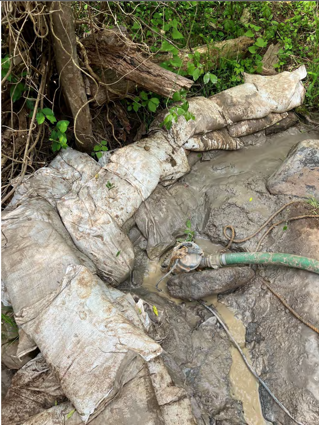
Figure D: Another of the frac-outs within the channel of the waterway (UT to Monocacy River, use class I-P waters) just downstream where the farm stream crossing is located; there was sediment deposited in the stream where the frac-out occurred. This frac-out is located at Segment 2. Sediment (bentonite) pollution is occurring in the Waters of the State but is contained in a portion of the waterway.
