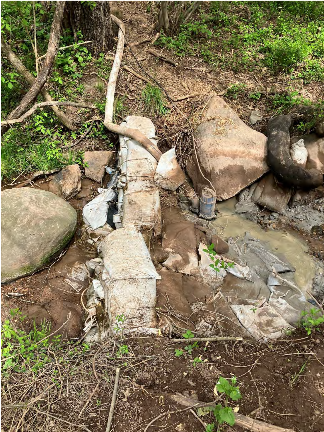
Figure B: The furthest upstream (UT to Monocacy River, use class I-P waters) frac-out is contained and previously documented. This frac-out is located at Segment 2. Sediment (bentonite) pollution is occurring in the Waters of the State but is contained in a portion of the waterway.
