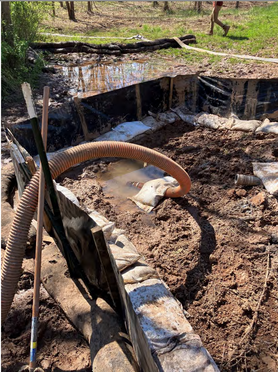
Figure E: There was a frac-out on the western side of the waterway (UT to Monocacy River, use class I-P waters), this frac-out was on dry land and contained with filter logs, sandbags, and silt fence. Sediment (bentonite) pollution was found in the Waters of the State and remains in a condition likely to continue to pollute. There was substantial sediment (bentonite) pollution downstream of where the frac-outs were located.
