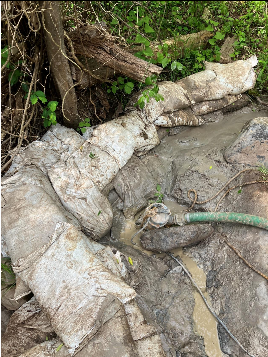
Figure D: Another of the frac-outs within the channel of the waterway (UT to Monocacy River, use class I-P waters) just downstream where the farm stream crossing is located; there was sediment deposition deposited in the stream where the frac-out occurred. This frac-out is located at Segment 2. Sediment (bentonite) pollution is occurring in the Waters of the State but is contained in a portion of the waterway.
