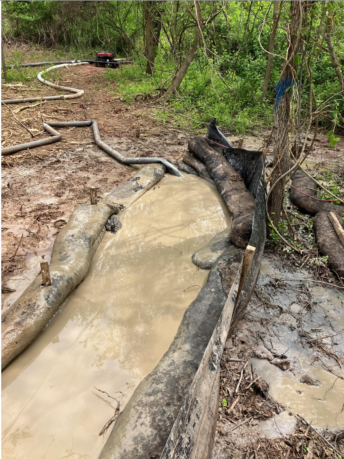
Figure A: One of the undocumented frac-outs was found by the documented (in the 04/10/2024 MDE inspection report) frac-out on the western side of the waterway (UT to Monocacy River, use class I-P waters), on dry land. This frac-out is located at Segment 2. Sediment (bentonite) pollution is occurring in the Waters of the State but is contained at a downstream point.
