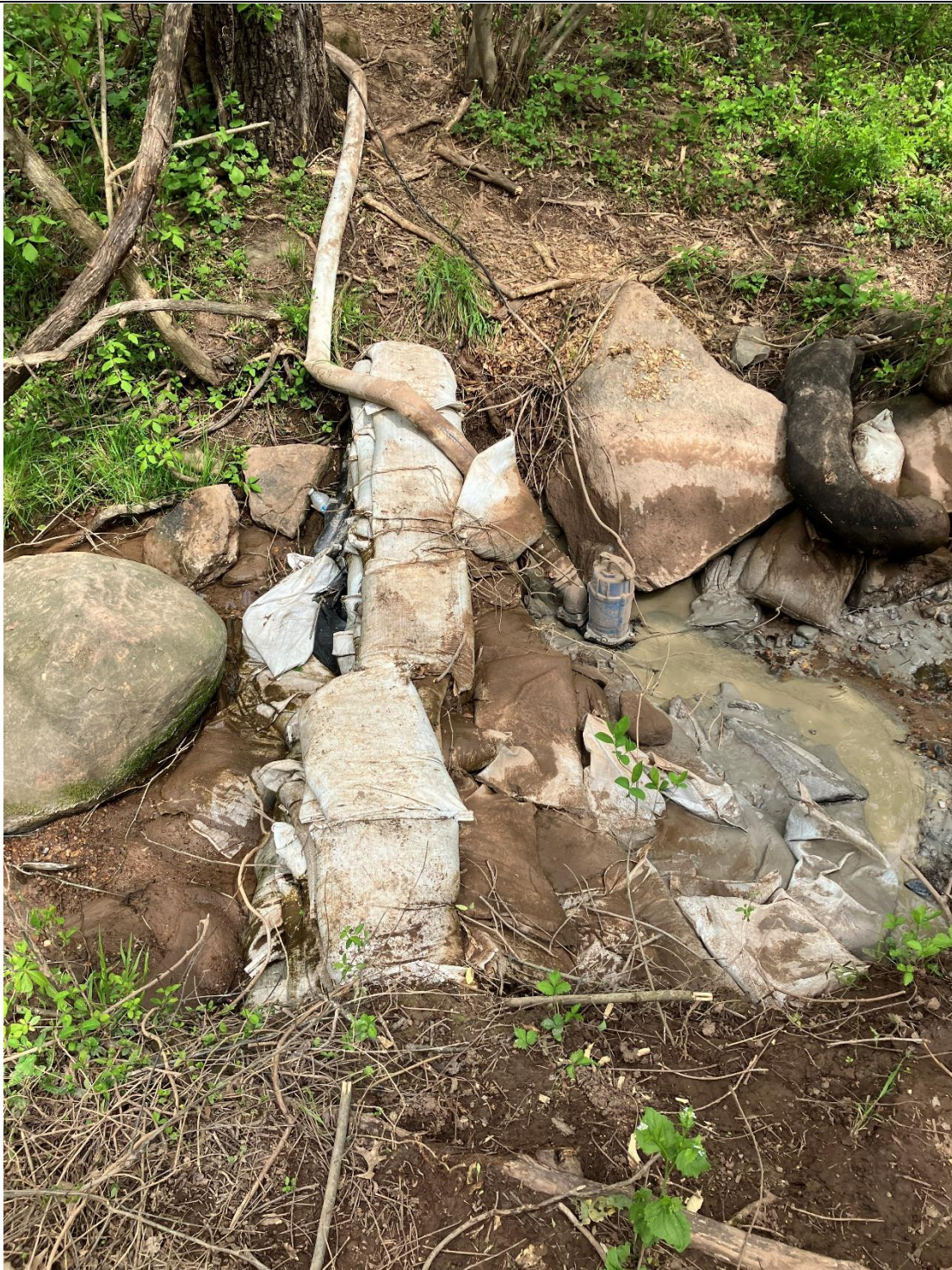
Figure B: The furthest upstream (UT to Monocacy River, use class I-P waters) frac-out is contained and previously documented. This frac-out is located at Segment 2. Sediment (bentonite) pollution is occurring in the Waters of the State but is contained in a portion of the waterway.
