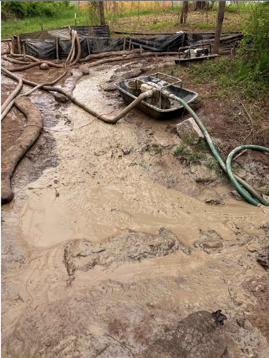
Figure E: The two frac-outs on the western bank of UT to Monocacy River are discharging into the waterway and are not individually contained. These frac-outs are located at Segment 2. The one frac-out is the same one documented in Figure A. Sediment (bentonite) pollution is occurring in the Waters of the State but is contained at a downstream point.
