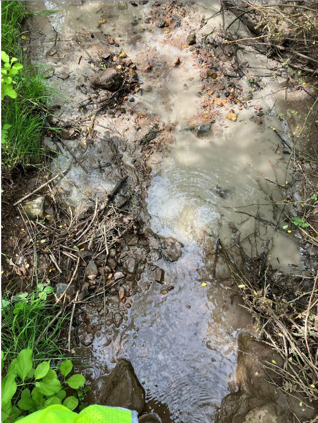
Figure C: The other undocumented frac-out was within the stream (UT to Monocacy River, use class I-P waters) channel just downstream of the documented (in the 04/10/2024 MDE inspection report) frac-out (frac-out in Figure B) that was contained with sandbags around the discharge point. This frac-out is located at Segment 2. Sediment (bentonite) pollution is occurring in the Waters of the State but is contained at a downstream point.
