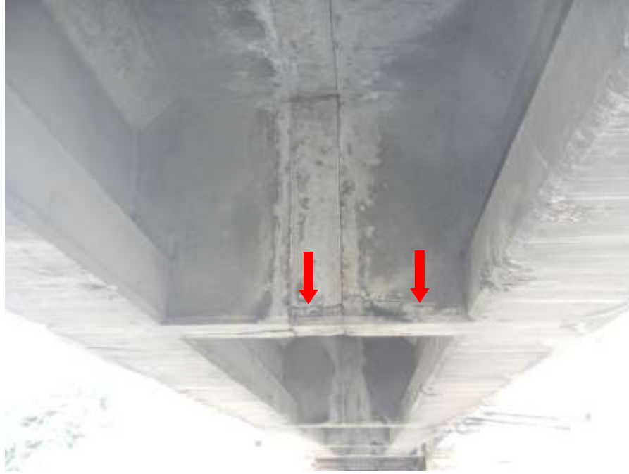
Photograph No. 29 – Crack in Underside of Third Diaphragm From East Abutment (Looking West)
