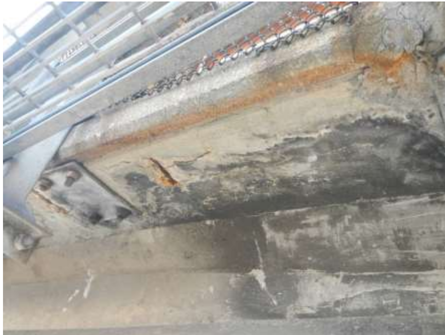
Photograph No. 22 – Area of Delaminated Concrete on North Deck Overhang Above Left Edge of Right Southbound Lane
