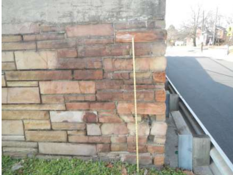
Photograph No. 41 – Area of Cracked and Missing Stones at Base of Wall Between North Ends of Northwest and Northeast Wingwalls (Looking South)
