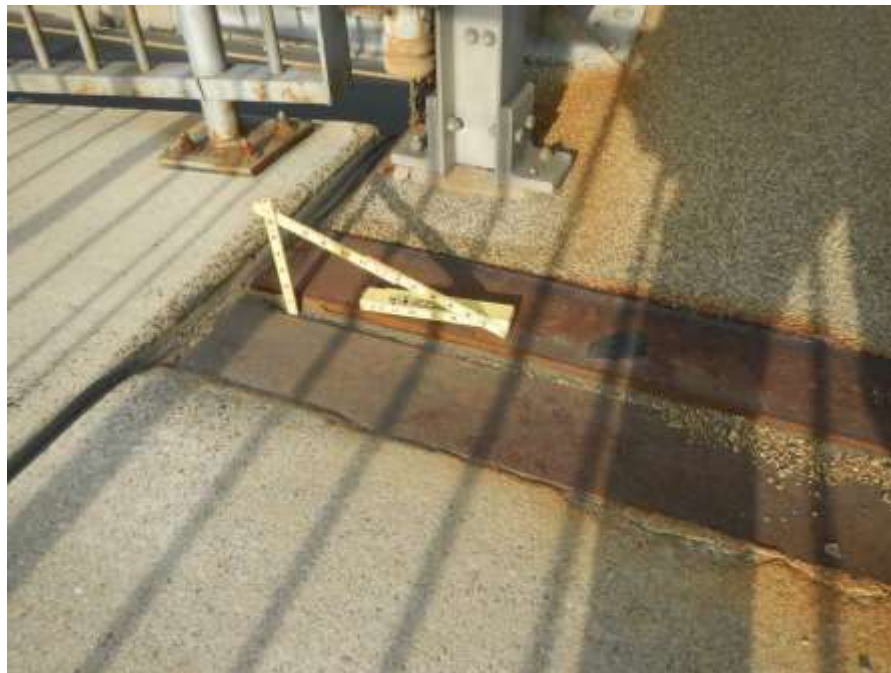
Photograph No. 16 – East Abutment Compression Joint Seal: East Side (Approach) Joint Armor Settled 1" at South End (Looking Southwest)
