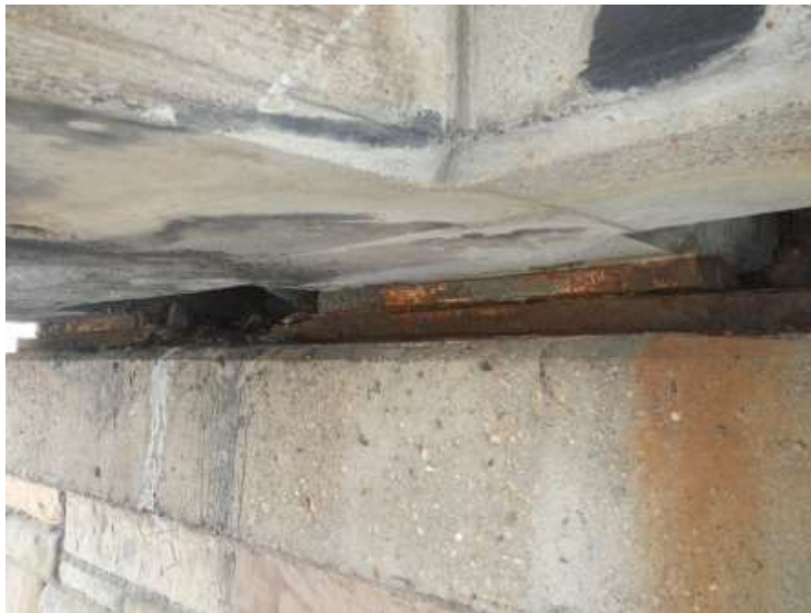
Photograph No. 32 – Steel Plate Fixed Bearings at East Abutment (Looking Northeast): Note Moderate Corrosion on Bearings
