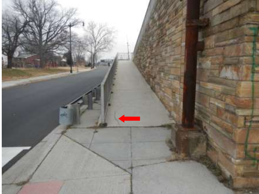
Photograph No. 3 – Lower Northwest Approach Pedestrian Ramp (Looking North): Note Portion of Full-Length Longitudinal Crack with Water Stains in Walking Surface
