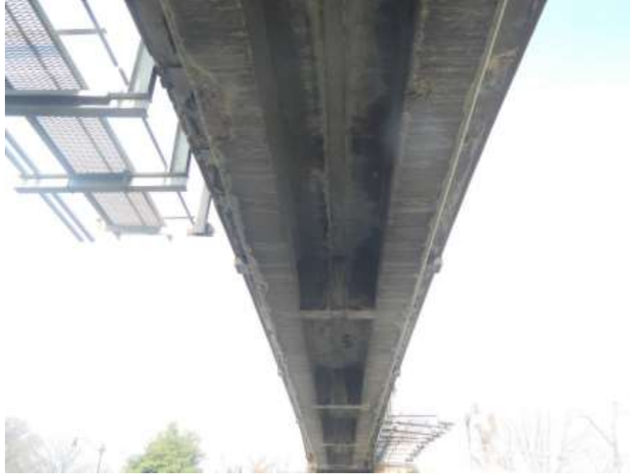
Photograph No. 19 – Typical View of Concrete Soffit/Underside of T-Beam Top Flange and Underside of Concrete T-Beams (Looking West): Note Prior Water Leakage Stains and Efflorescence Throughout Soffit
