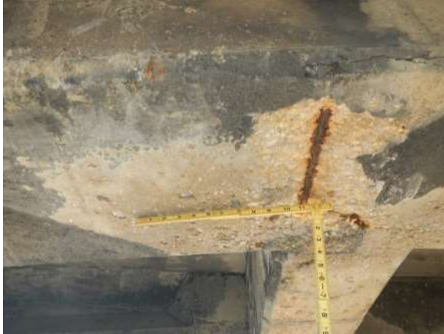
Photograph No. 27 – North T-Beam Underside at First Intermediate Diaphragm From West Abutment Above Right Southbound Lane: Spall with Exposed Corroded Reinforcing Steel (Looking South)
