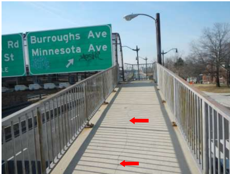
Photograph No. 4 – Upper Northwest Approach Pedestrian Ramp (Looking South): Note Portion of Full-Length Longitudinal Crack in Walking Surface
