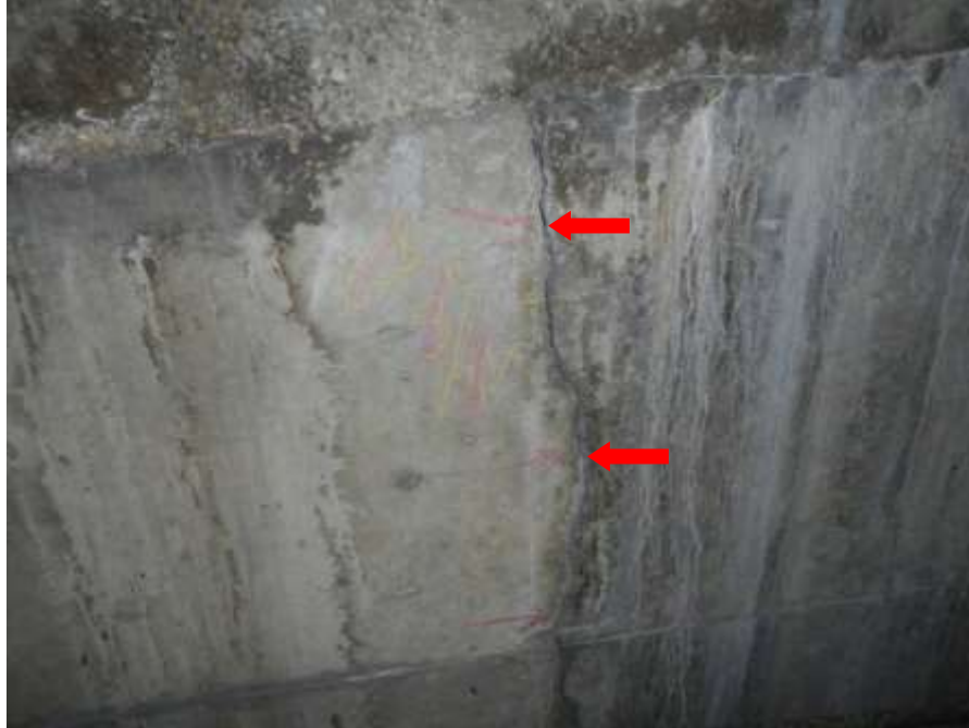
Photograph No. 35 – East Abutment Interior: Vertical Crack in East and West Faces of Concrete Interior Wall Between Approach Ramps at Approximately One-Third Point From South End (West Face Shown, Looking East)
