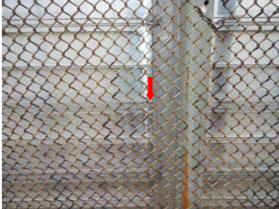
Photograph No. 47 – Right/West Overhead Directional Sign on North Side of Bridge: Third Sign Clip From Bottom Missing on Second Vertical Attachment Member From West (Looking North)
