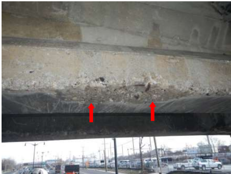
Photograph No. 28 – South T-beam Above Right Northbound Lane (Looking North): Spall with Exposed Corroded Reinforcing Steel on South Edge and Underside
