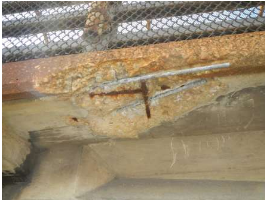
Photograph No. 20 – Spall with Exposed Corroded Reinforcing Steel Near East End of North Deck Overhang Above Right Northbound Lane (Looking South)
