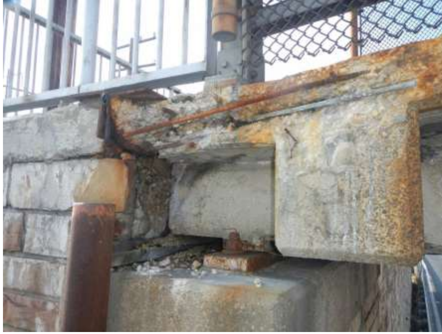
Photograph No. 21 – Spall with Exposed Corroded Reinforcing Steel at Northeast Corner of Deck Fascia/Overhang Under First Safety Fence Post (Looking Southeast)
