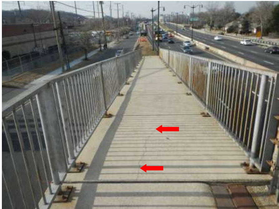
Photograph No. 8 – Upper Southeast Approach Pedestrian Ramp (Looking South): Note Portion of Full-Length Longitudinal Crack in Walking Surface
