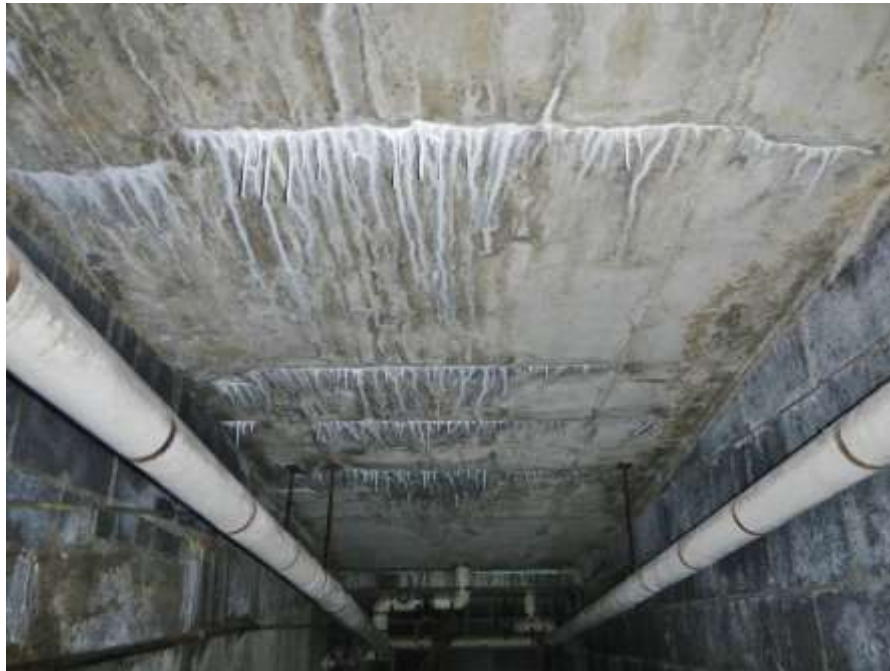
Photograph No. 44 – West Abutment Interior, Underside of Upper Northwest Approach Pedestrian Ramp: Water Stains with Moderate Efflorescence and Stalactites
