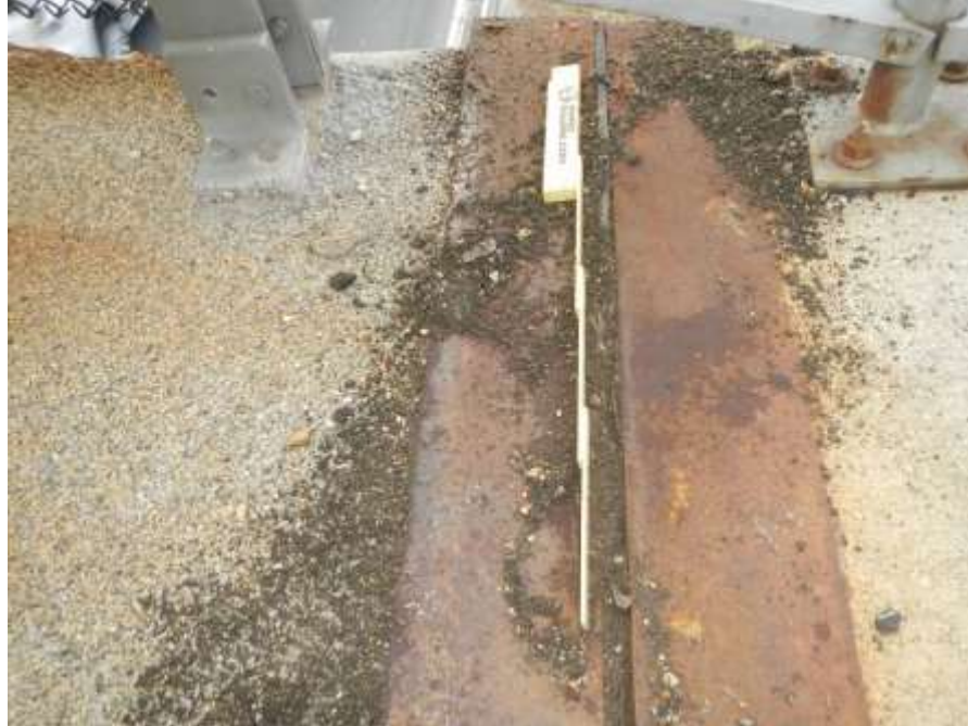
Photograph No. 15 – West Abutment Compression Joint Seal Debonded From West Joint Armor at South End (Looking South)
