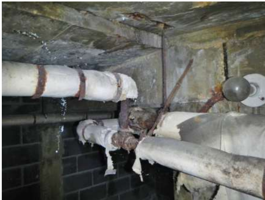
Photograph No. 52 – Two Broken Supports for Pipes of Non-Functional Antifreeze System at North End of Lower Pedestrian Approach Ramp Inside West Abutment
