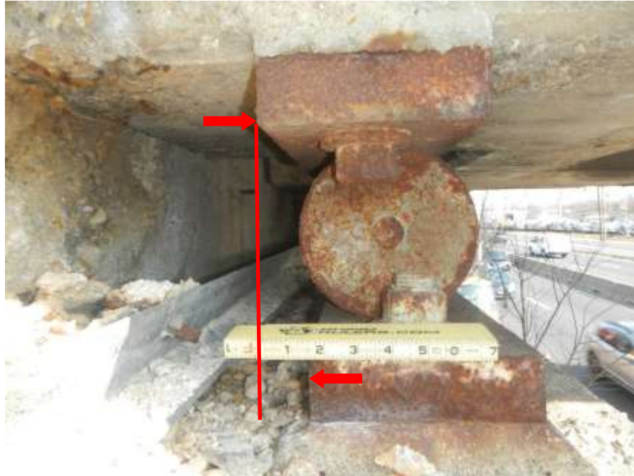
Photograph No. 31 – Steel Roller Expansion Bearings at West Abutment 1½" in Expanded Position Measured at Ambient Temperature of 46° Fahrenheit (South Bearing Shown, Looking North)
