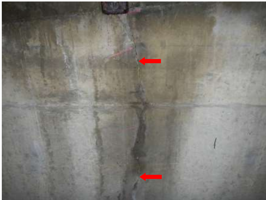
Photograph No. 40 – West Abutment Interior: Vertical Crack in East and West Faces of Concrete Interior Wall Between Upper and Lower Pedestrian Approach Ramps 18 Ft. From North End (East Face Shown)
