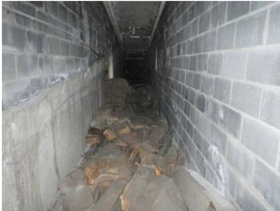
Photograph No. 36 – East Abutment Interior: Significant Accumulation of Debris on Concrete Floor Under Upper Pedestrian Approach Ramp From Just Beyond Utility Room Extending to South End of Ramp (Looking South)
