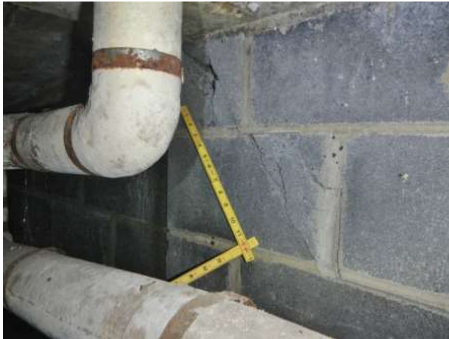
Photograph No. 38 – West Abutment Interior: Area of Cracked and Broken Cinderblocks at Top of East/Interior Face of Cinderblock Wall at Northwest Wingwall Near North End
