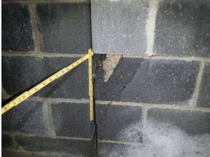
Photograph No. 39 – West Abutment Interior: Diagonal Crack with Adjacent Spall Near Base of East/Interior Face of Cinderblock Wall at Northwest Wingwall Near North End (Looking West)
