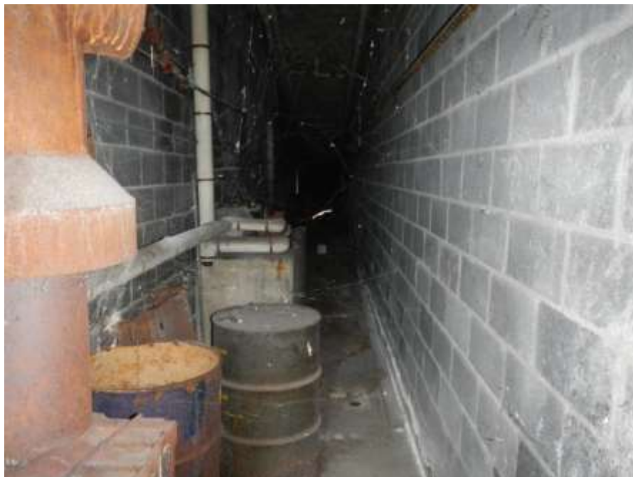
Photograph No. 34 – View Inside East Abutment Under Upper Pedestrian Approach Ramp (Looking South From Access Door)
