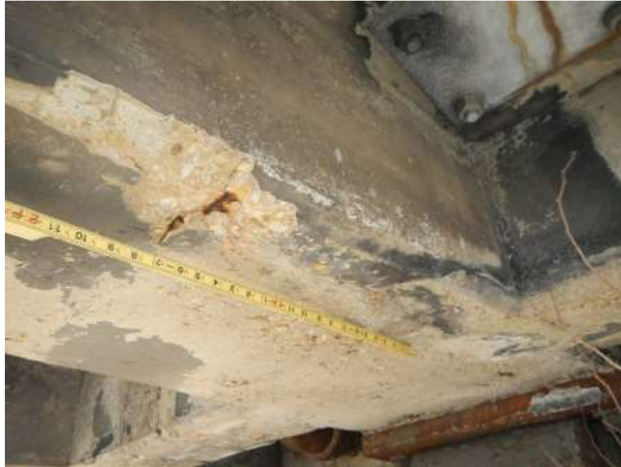
Photograph No. 25 – North T-Beam Underside Adjacent to End Diaphragm at West Abutment: Area of Delaminated Concrete and Spall with Exposed Corroded Reinforcing Steel (Looking Southwest)
