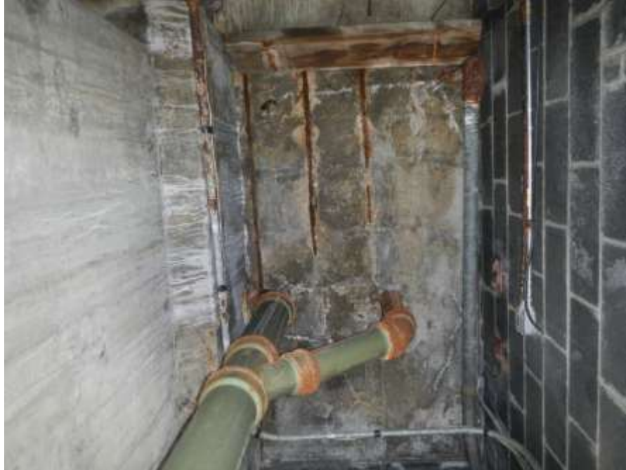
Photograph No. 43 – West Abutment Interior, Underside of Upper Northwest Approach Pedestrian Ramp: Intermittent Spalls with Exposed Corroded Reinforcing Steel Bars Near Access Door
