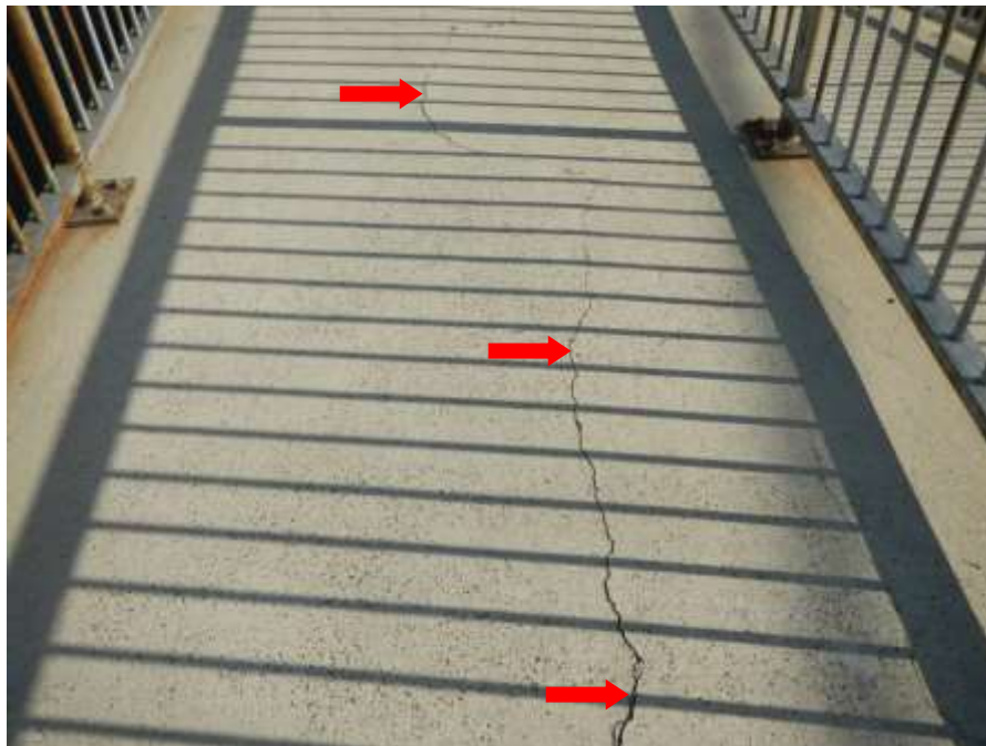
Photograph No. 42 – Full-Length Longitudinal Crack in Walking Surface of Upper Southeast Approach Pedestrian Ramp (Looking North)
