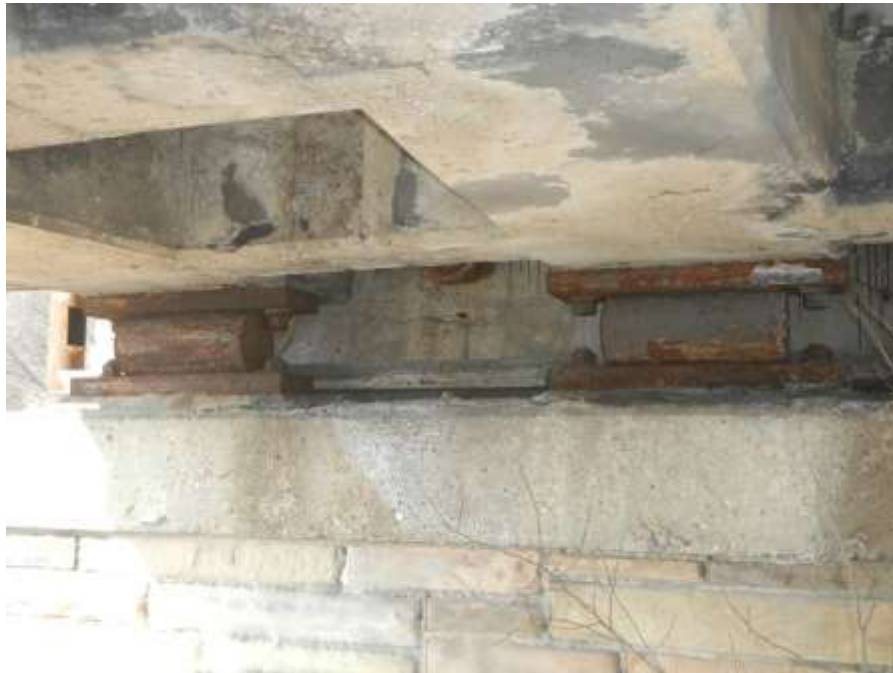
Photograph No. 30 – Steel Roller Expansion Bearings at West Abutment: Note Minor to Moderate Corrosion on Bearings
