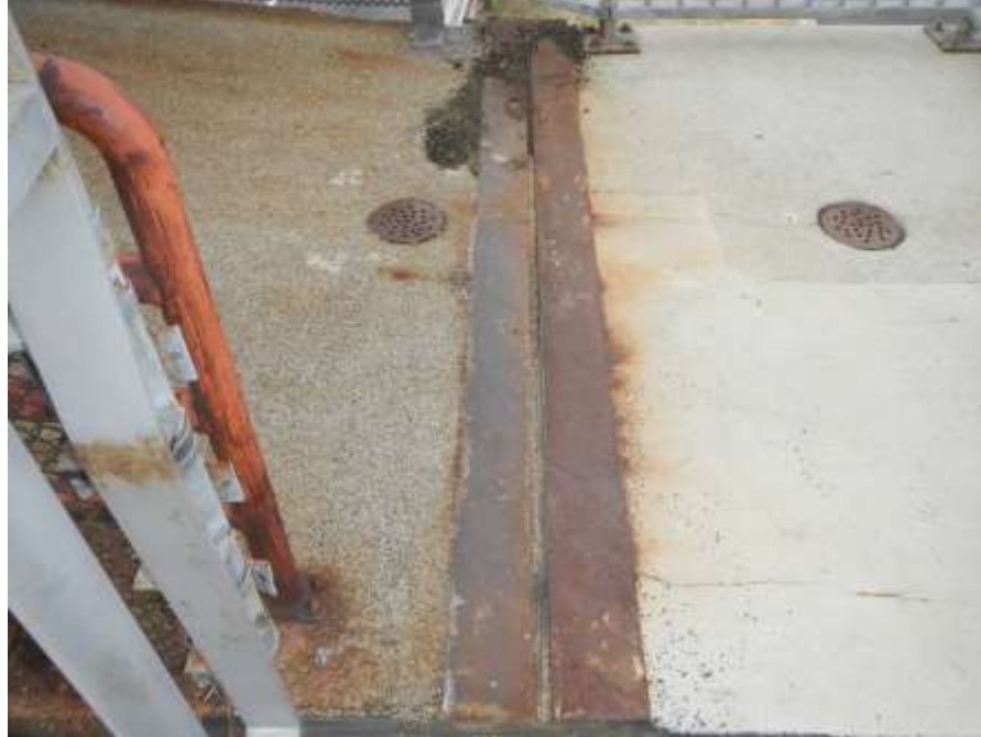
Photograph No. 13 – Typical Compression Joint Seal (West Abutment Shown, Looking South): Note Corrosion on Joint Armor
