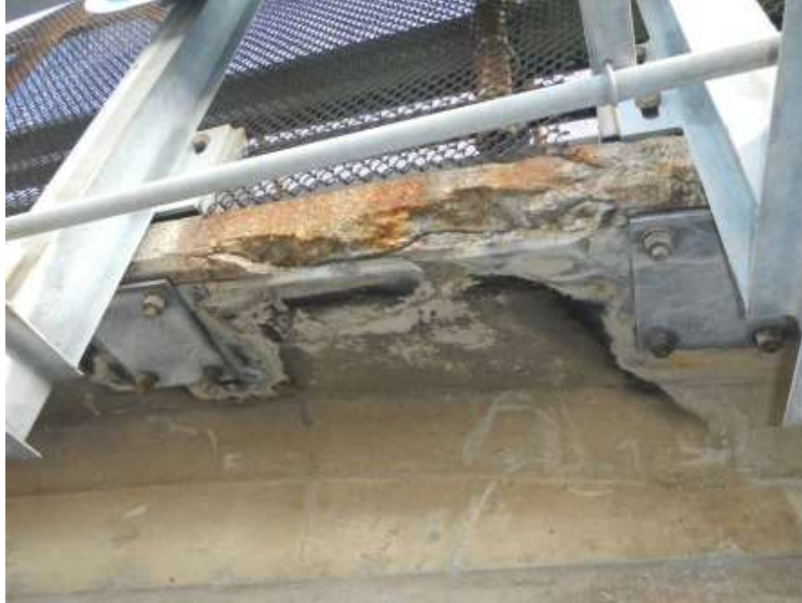
Photograph No. 23 – Area of Delaminated and Loose Concrete on South Deck Fascia/Overhang Above Lane Striping Between Right and Center Northbound Lanes of Kenilworth Avenue (Looking North)
