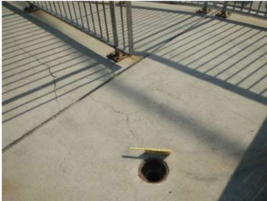
Photograph No. 46 – Missing Drainage Grate at South End of Upper Southeast Approach Ramp (Looking Northeast)
