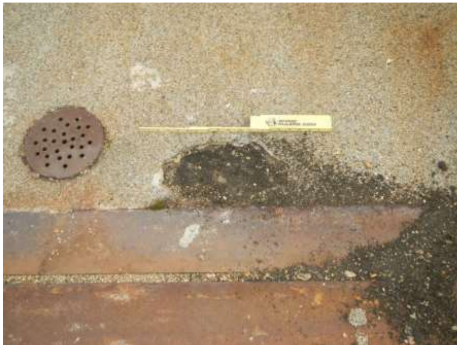
Photograph No. 12 – Spall in Deck Wearing Surface Adjacent to West Abutment Joint (Looking East)
