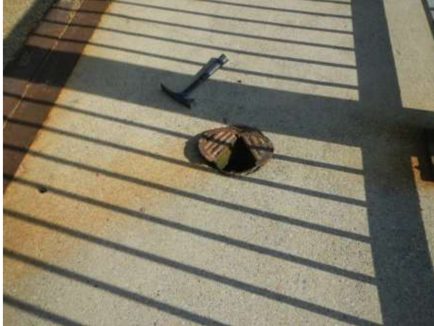
Photograph No. 45 – Cracked/Broken/Loose Drainage Grate at North End of Upper Southeast Approach Ramp: Note Concrete Debris Blocking Six of Eight Openings in Grate (Looking North)
