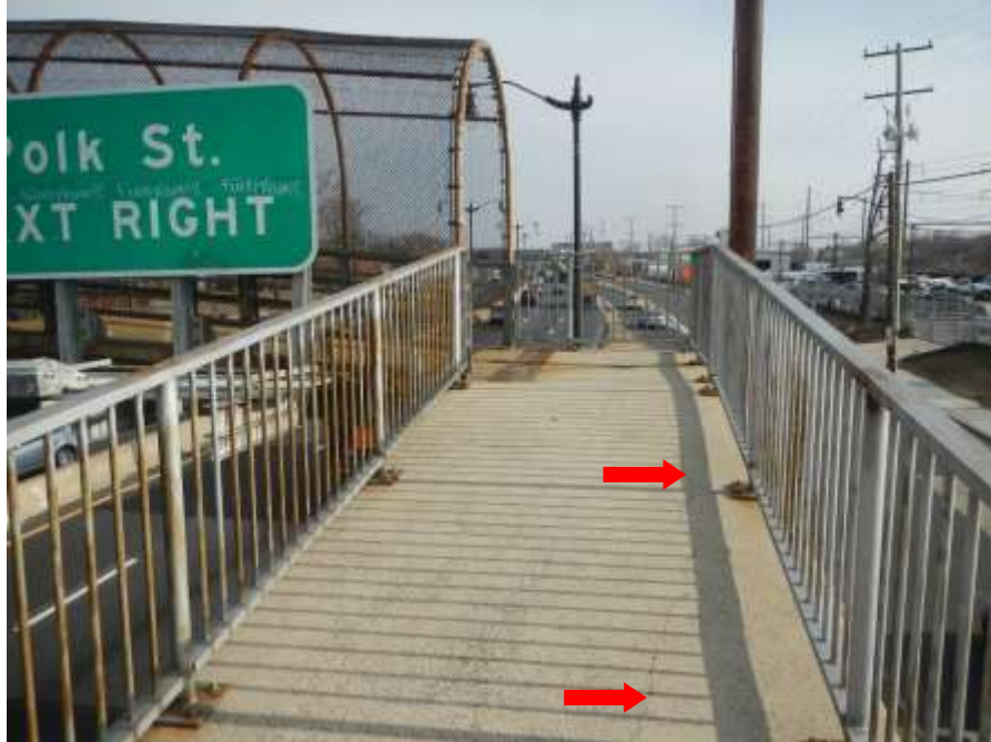
Photograph No. 7 – Upper Southeast Approach Pedestrian Ramp (Looking North): Note Portion of Full-Length Longitudinal Crack in Walking Surface
