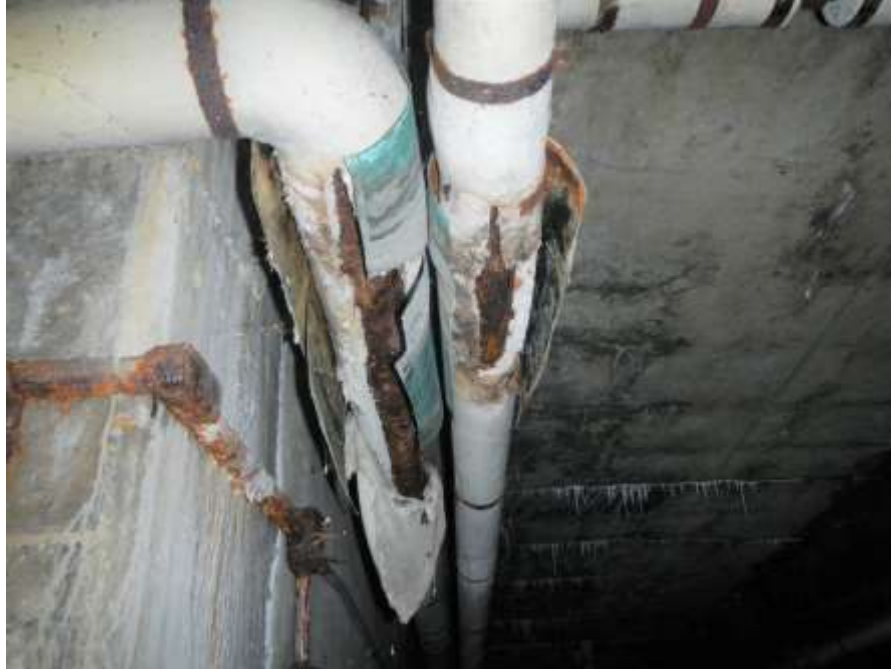
Photograph No. 51 – Severe Corrosion and Pipe Wrapping Unraveled on Two Pipes of Non-Functional Antifreeze System at South End of Lower Pedestrian Approach Ramp Inside East Abutment
