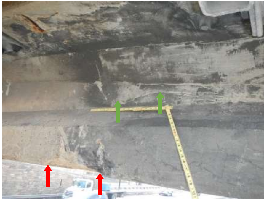
Photograph No. 26 – North T-beam Above Right Southbound Lane (Looking South): Spall on North Edge and Underside (Red Arrows); Horizontal Crack in North Face Web (Green Arrows)
