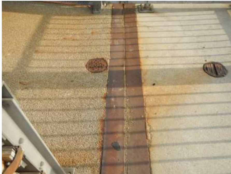
Photograph No. 14 – Typical Compression Joint Seal (East Abutment Shown, Looking North): Note Corrosion on Joint Armor
