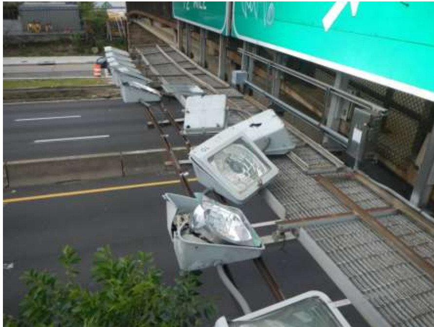
Photograph No. 50 – Damaged/Broken Lights for Directional Sign on North fascia Above Southbound Lanes of Kenilworth Avenue
