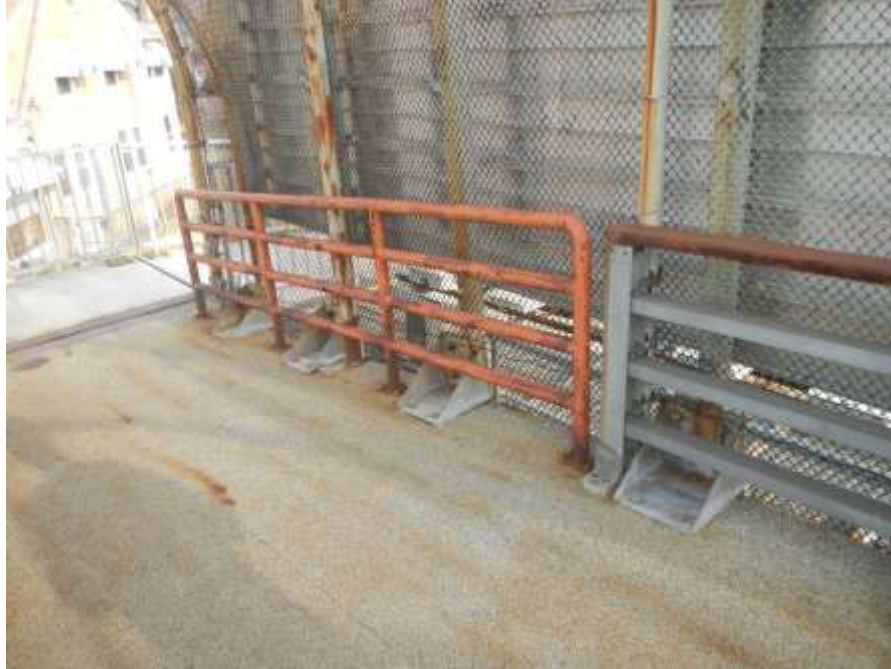
Photograph No. 17 – Non-Standard Tubular North Bridge Railing at West End (Looking Northwest)
