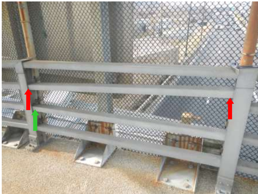
Photograph No. 18 – South Bridge Railing, Third Section from East: Both Connection Bolts Missing at Second Rail from Top – Rail Unsecured (Looking South): Note One Missing Connection Bolt at Third Rail from Top
