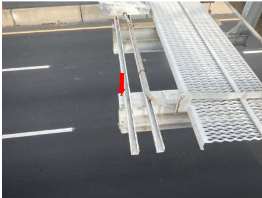
Photograph No. 48 – South and North Channels for Directional Sign Light Support on South Side of Bridge Disconnected at East End Due to Missing Bolts (Looking West)
