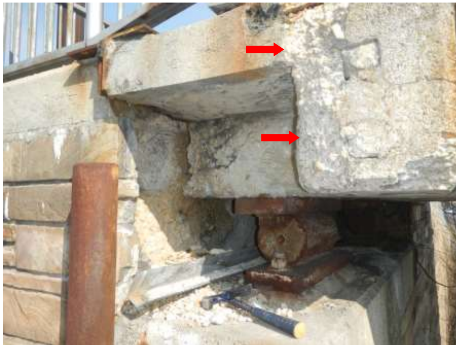
Photograph No. 24 – Spall with Exposed Corroded Reinforcing Steel in South Deck Fascia Near West Abutment (Looking Northwest)
