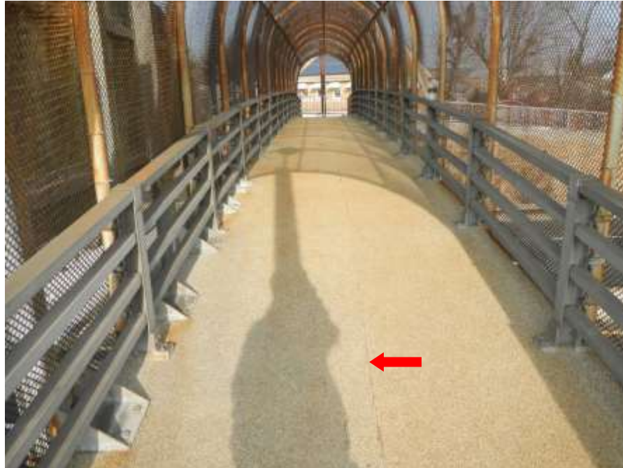
Photograph No. 11 – Typical Deck Wearing Surface, Steel Bridge Railings and Steel Arch Safety Fence (Looking West): Note Longitudinal Crack
